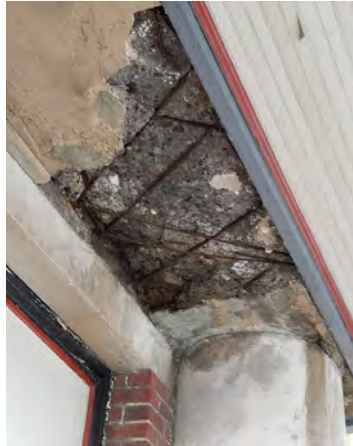
DAMAGED CANOPY AT COLUMN
