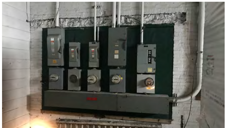
ELECTRICAL SERVICE STATION IN BAGGAGE/EXPRESS BUILDING
