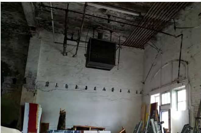
SUSPENDED GAS HEATER IN BAGGAGE/EXPRESS BUILDING
